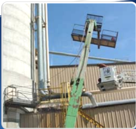
A welder in Iowa fell to his death from this platform attached to the forks of a boom forklift. The 4 X 12 platform was made by the company specifically for use with their rough terrain lift. The killed worker was 35-40 feet high when he fell, landing on a catwalk 20 feet below.
